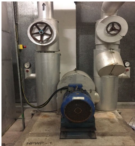
Photo A.12 Chilled water pump
