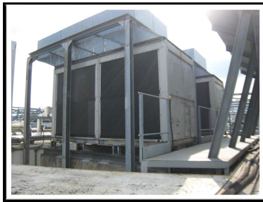
Photo A.11 Air cooled chiller
