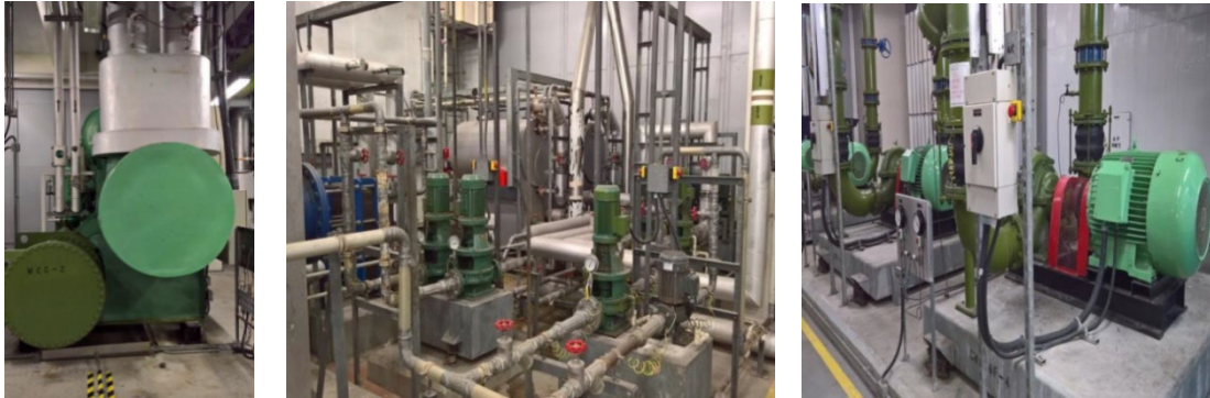
Photo A.20 Chiller plant equipments
