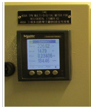
Photo A.15 A metering device for a 400A circuit
